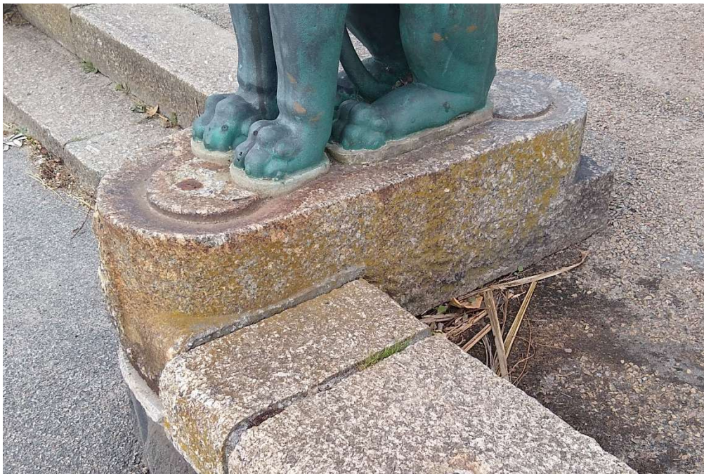
Loose Bedding, Pointing with Debris under stone
