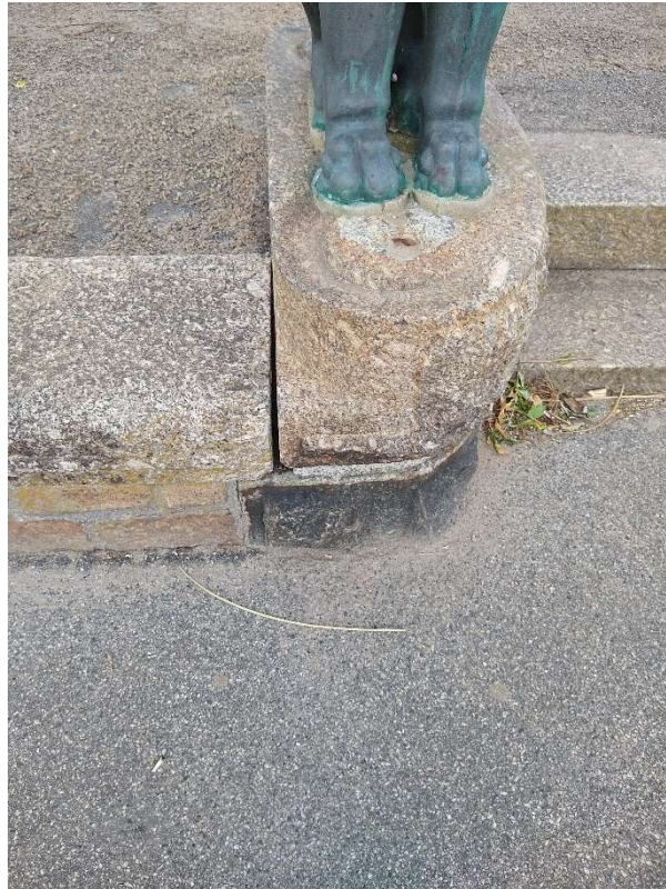
Displaced Capping Stone and Bedding
