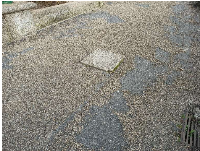
Raised access cover
