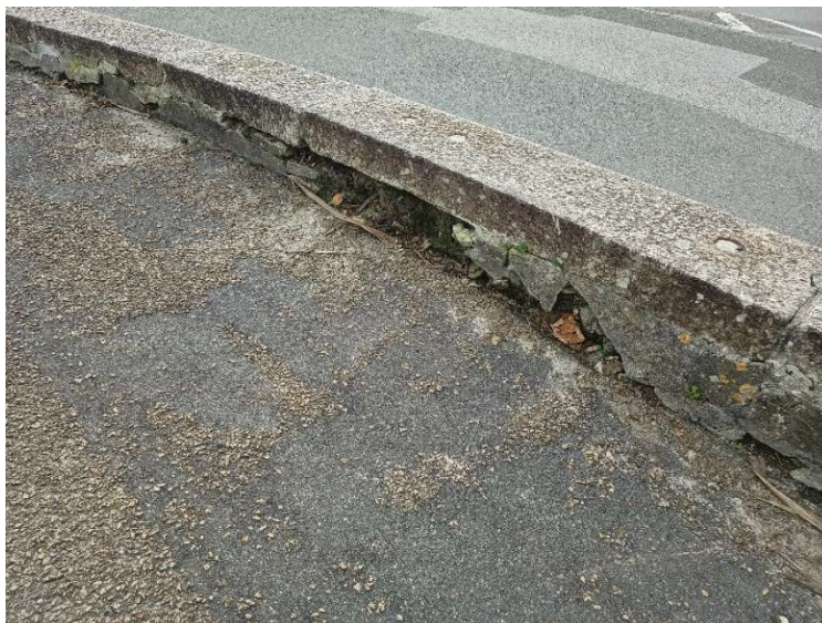
Mortar pointing/render displacement (2024)
