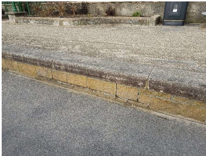
Terrace Edge with Failing Mortar (2024)
