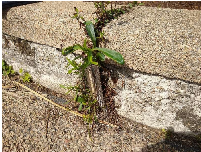
Failed Render and Exposed Beading / Weed Growth
