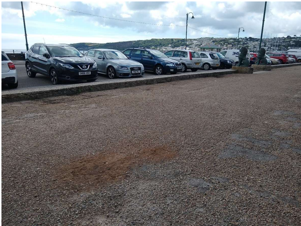
Visible hollows in surface against Terrace Edge
