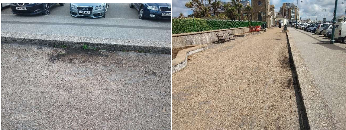
Areas of Pooling Water leaving debris
