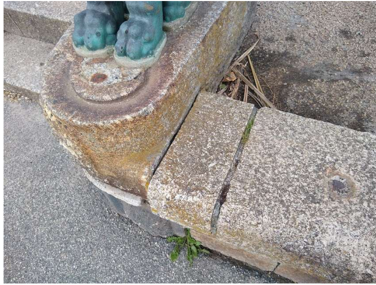
Loose Capping Stone
